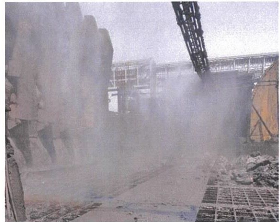
Fig: Dust suppression system in Wagon Tripler
