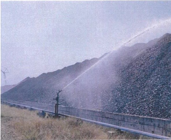
Fig: Dust suppression system in Coal yard
