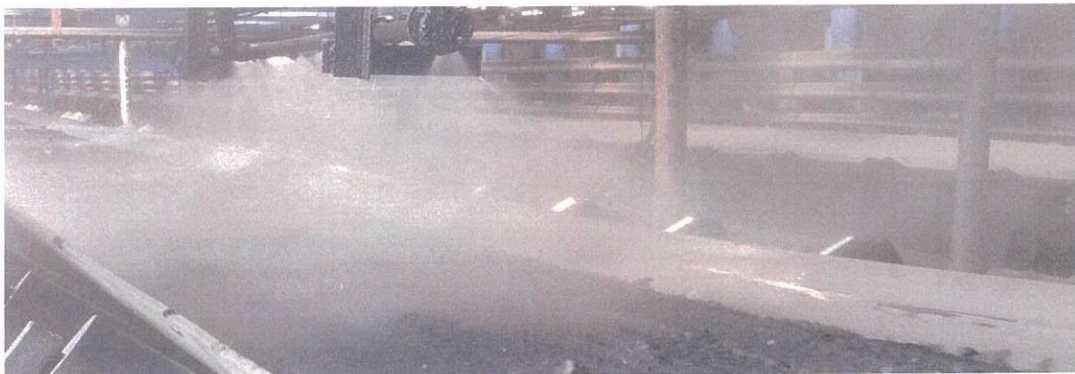
Fig: Dry Fog Dust suppression system in Conveyor belts
