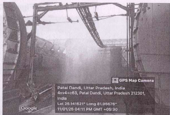
Figure: Water Sprinkling at Wagon Tippler
