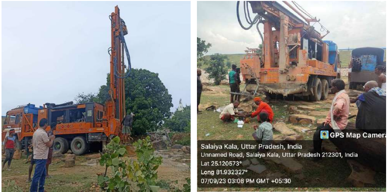
Figure 6.5: Drilling operation in progress for construction of the Piezometer around new Ash Dyke, NTPC Meja,
